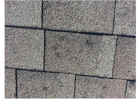
Common hail hits to an asphalt shingle
